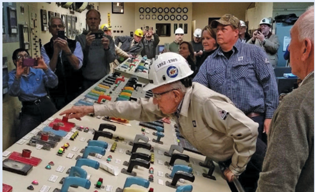
Retiree Mac Flowers opens breaker separating Johnsonville Fossil Plant's last unit from the TVA grid.
