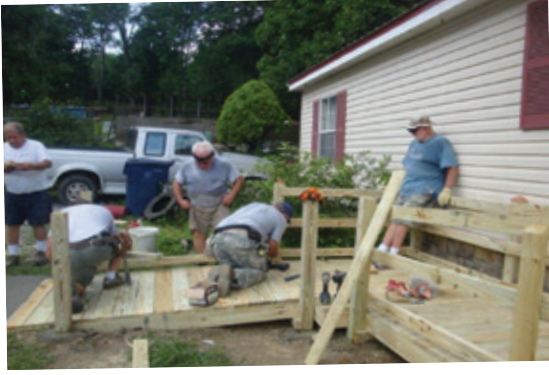
A ramp project nearing completion by Chattanooga Chapter retiree volunteers working along with others
