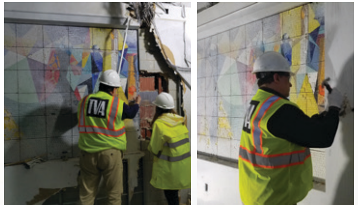
Workers carefully remove pieces of the Robert Birdwell mural at decommissioned Widows Creek Fossil Plant.
