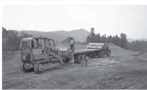
Early phase of construction of Thomas Village in 1978, a small residential development with energy-efficiency features designed by TVA to accommodate residents impacted by severe flooding at Clinchport, Va. “It’s a thriving little place now.”
