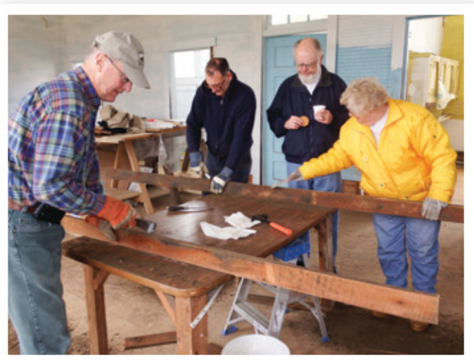
After almost five years of major restoration, the Oak Grove School is one of the completed projects sponsored by the Knoxville Chapter.
